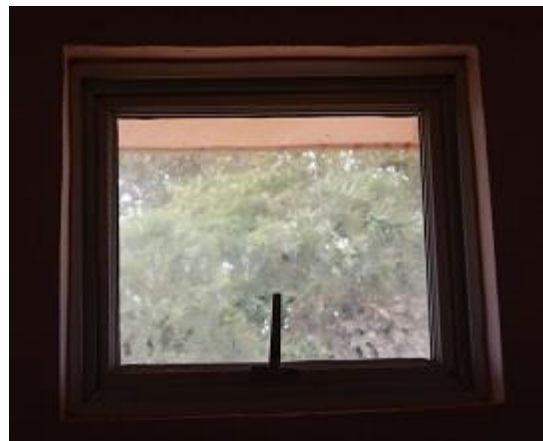
Pic: Window which is not properly aligned
